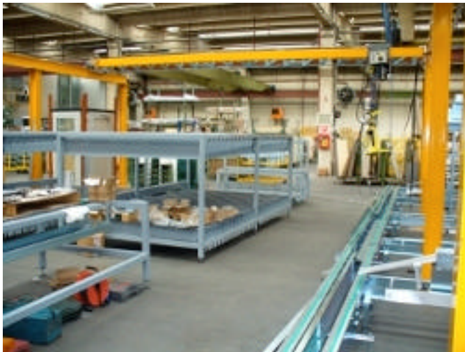
Front view of the bridge crane
